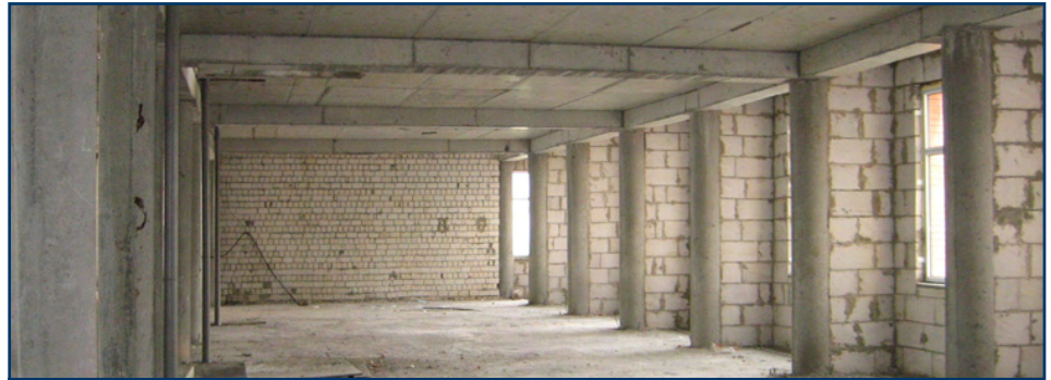
Though the expansion looks finished from the outside, its sparse, concrete-block rooms still need lots of work before students can move in.
